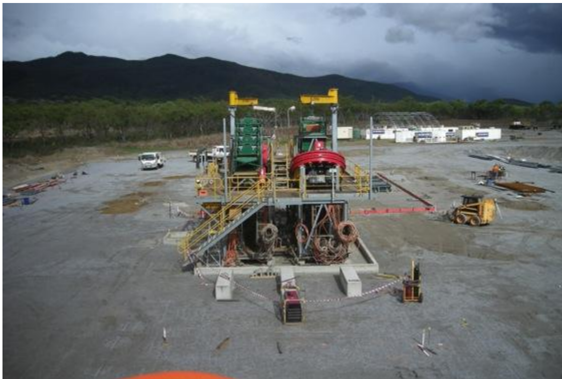
The Kelsey Jig Relocatable Processing Plant showing the concrete "plinths" for the MCC.
