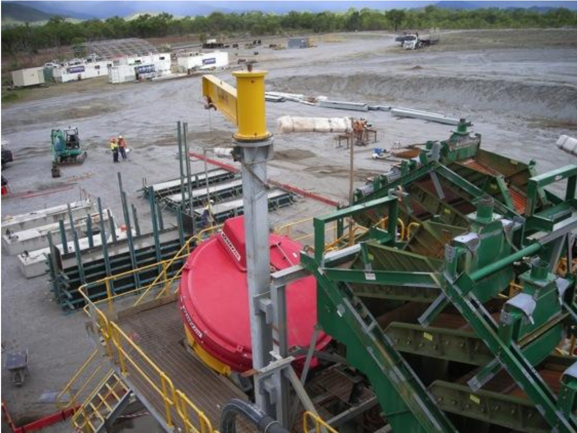
The Kelsey Jig Relocatable Processing Plant installed and complete showing the view back towards the shaking table foundations.
