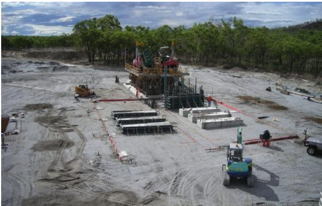
Tailings Re-Treatment Processing Plant Construction showing the fully completed Kelsey Jig Processing Plant and Concrete Foundations for the Shaking Table Concentrate Circuit.
